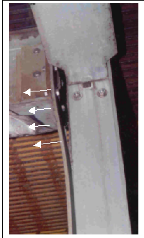
Figure 1. A Premature Local Failure of the Web/Flange Junction of Thin-walled E-glass/Polyester Pultruded Composite Column Exposed to Harsh Environments 4 . (Mosallam 1998) 4
